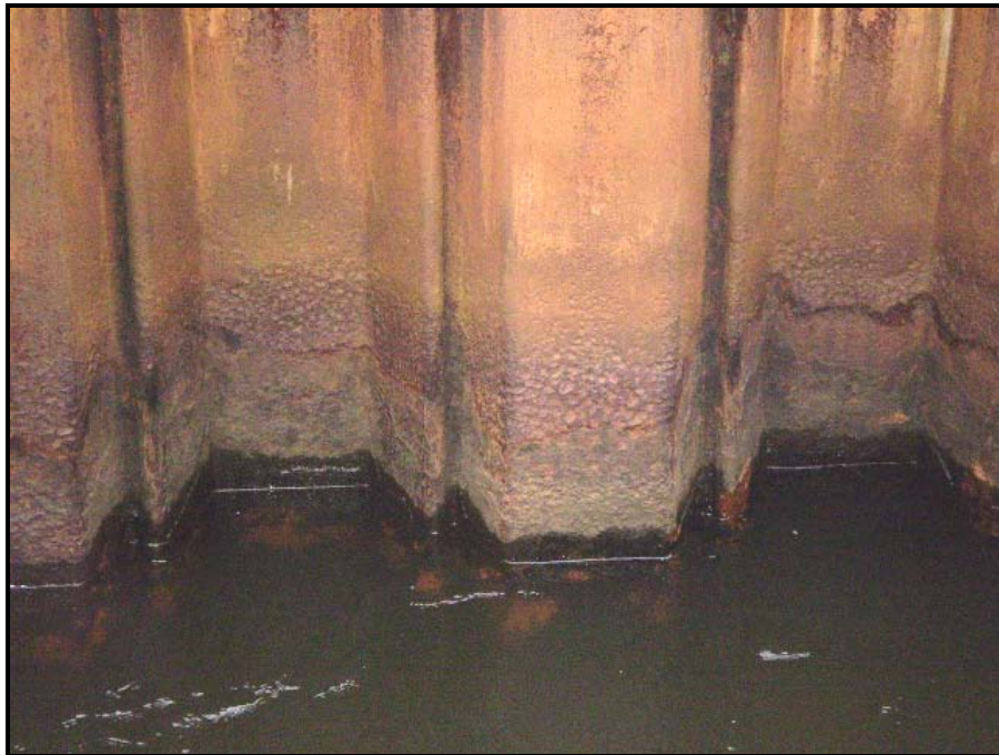
Photo 12 Typical Pitting at Waterline in Steel Sheet Pile Weir Wall
