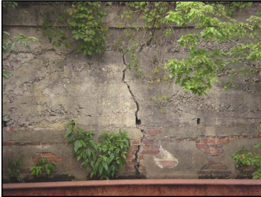
Photo 7 Vertical Crack in North Headwall, Also Note Heavy Honeycombing
