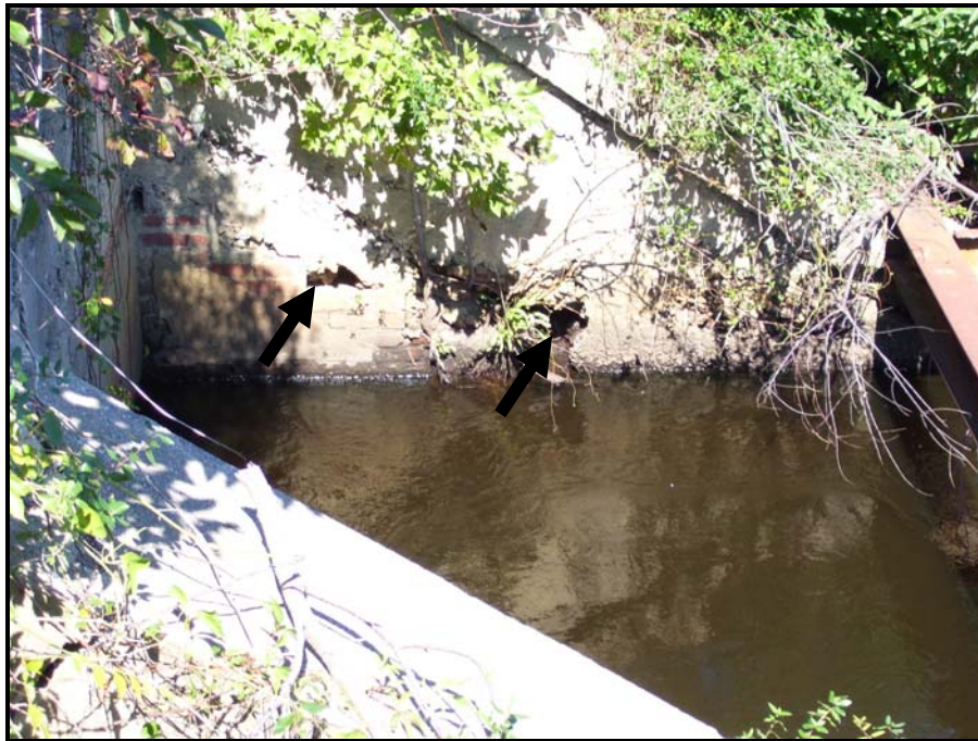
Photo 8 Voids in Northwest Wingwall at Masonry to Concrete Transition
