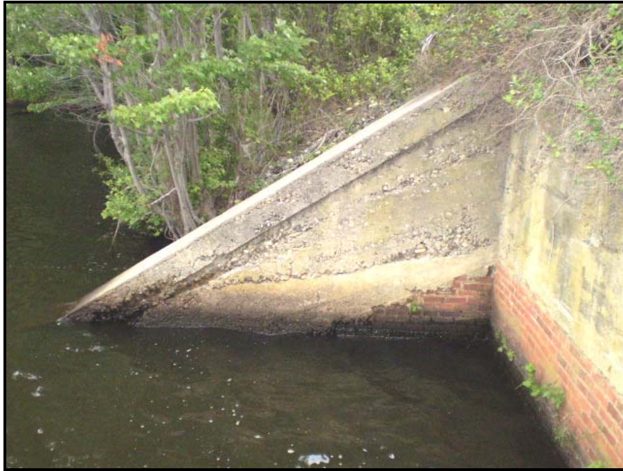
Photo 9 Elevation of Southwest Wingwall, Note Heavy Honeycombing
