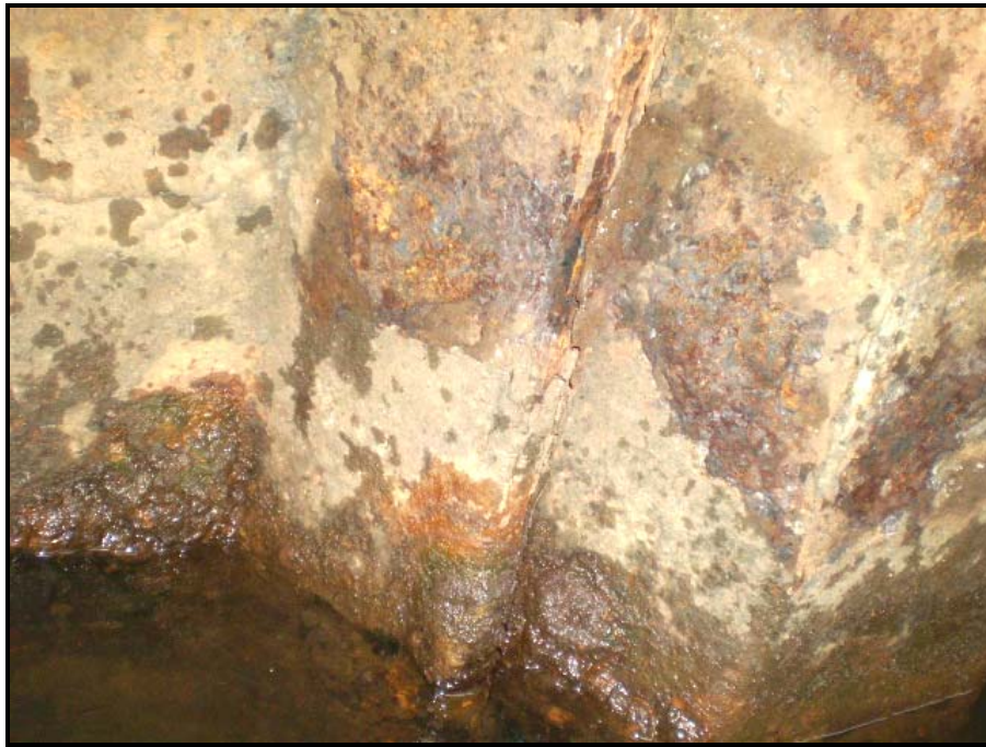
Photo 13 Typical Pitting at Waterline in Steel Sheet Pile Weir Wall
